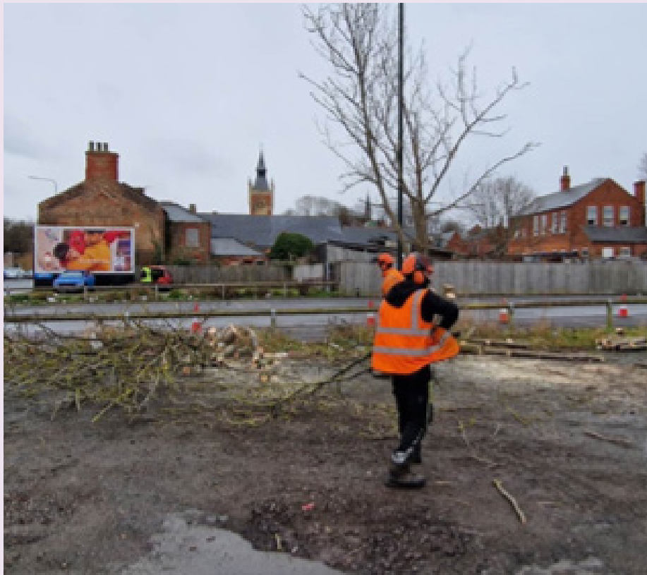
Wellington Street Car Park - removed wild trees and overgrown foliage prior to new permanent CCTV installation (high-risk VAWG area). Three new lighting installations, and new lampposts supporting the new CCTV network.
